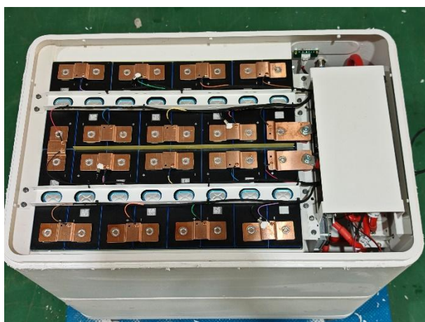
No.5.5-9 Inspection after test (Upper cavity)
