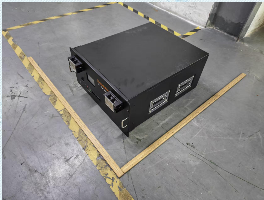
Figure 2 Overview of battery
